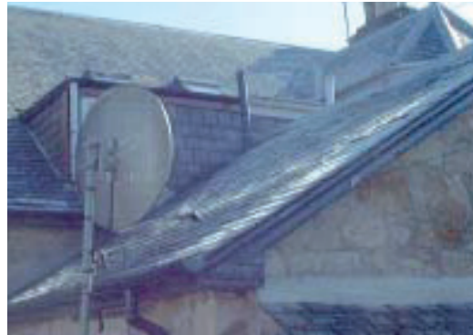
Good example of dish on building.
