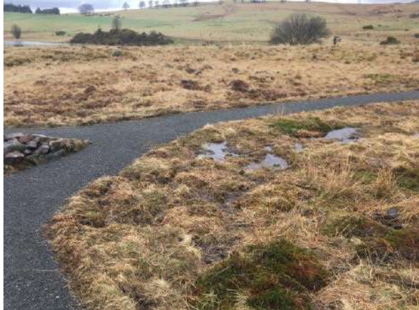
Location of standing water to be managed through additional culvert installation.
