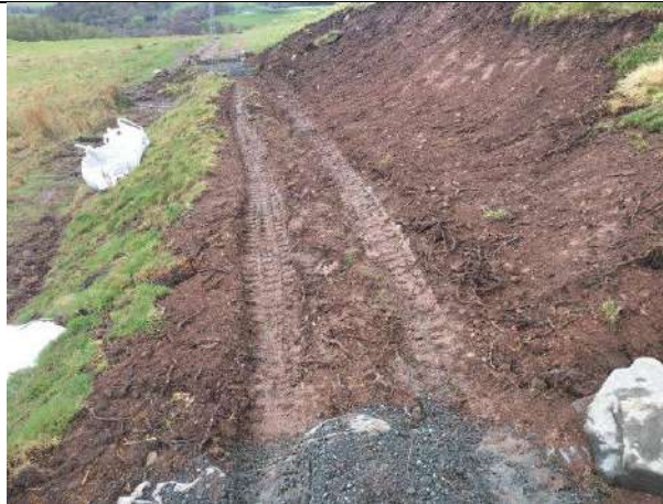
16.4 Section of steep slope which will be difficult to revegetate.
