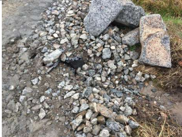
16.2 Damaged culvert near Cocksburn compound.
